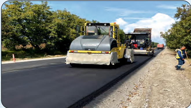
Moldova: Road Rehabilitation Project-IV (83Km), EBRD funded Scope: Construction Supervision under FIDIC Conditions of Contract
