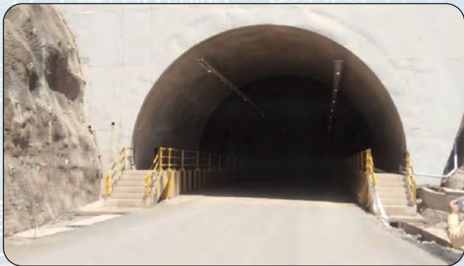
India: NH-22, Shimla Bypass, Kaithlighat-Dhalli Section (Twin Tube Tunnels, Total Length -5.292Km) Scope: Feasibility Study & Detailed Design
