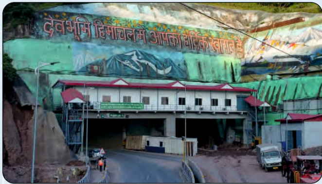
India: NH-21 Kiratpur to Nerchowk Section (Single Tube Tunnels, Total Length-4.820Km) Scope: Independent Engineer for Construction Supervision
