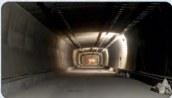
India: Z-Morh Tunnel (Length-6.412Km) Single Tube Bi-Directional Tunnel Scope: Independent Engineer for Construction Supervision
