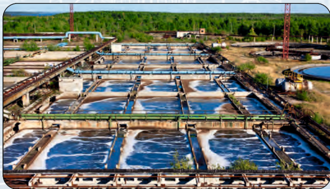
India: Multi Sector Infrastructure Rehabilitation Project (DSC-II), ADB funded Scope: Design & Construction Supervision
