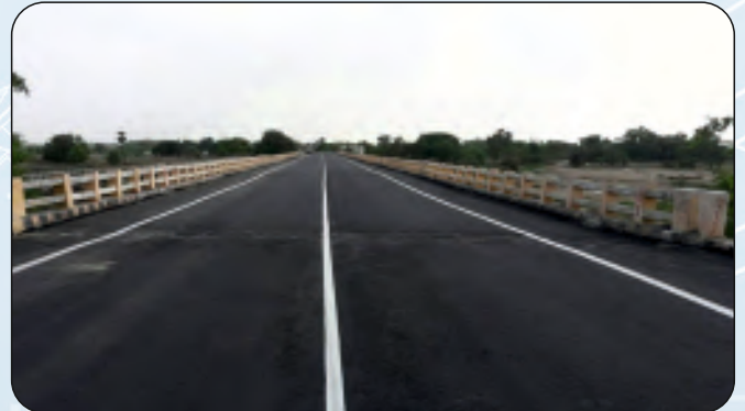
India: NH-98, Anisabad Aurangabad Hariharganj Section (154.625Km), World Bank funded Scope: Construction Supervision under FIDIC Conditions of Contract including Performance Based Maintenance
