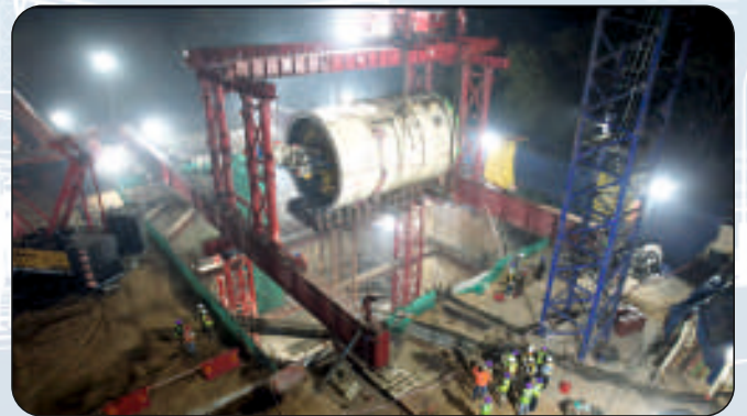
India: Aerocity to Tughlakabad Corridor Phase-IV Delhi MRTS, DC-09 Scope: Detailed Design including 5Km Twin Tube TBM Tunnel
