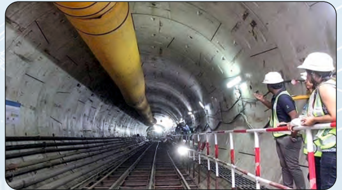
India: Mumbai Metro Line-3, Underground Corridor (UGC-03) (TBM Tunnel of Total Length-7.57Km) Scope: Detailed Design & Design Support during Construction
